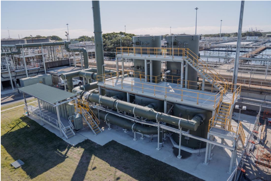
Figure 1 Air Treatment Facility (Inlet Works in the background to the left)
